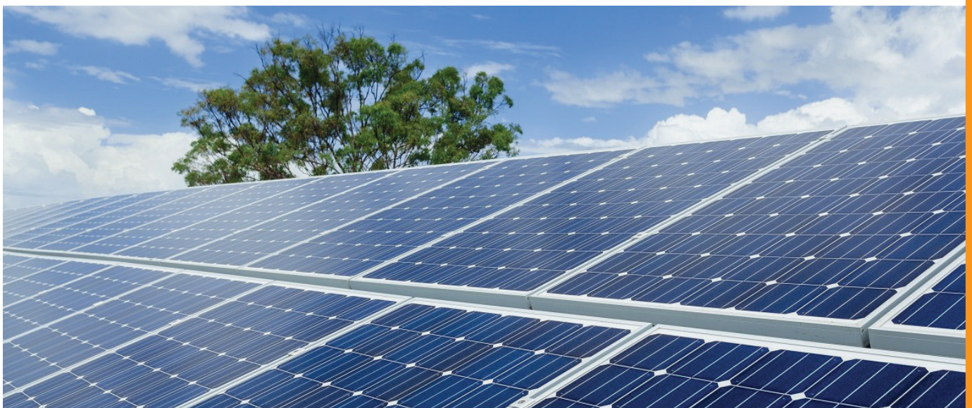
PHOTO VOLTAIC CABLE (SOLAR)
